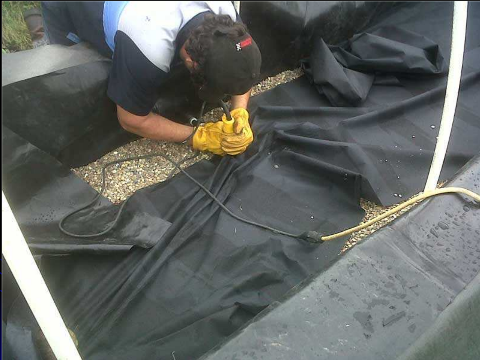
Another view of the drain hole
